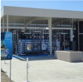
Potable Water Reuse & Purple Pipe Hundreds of Millions $
